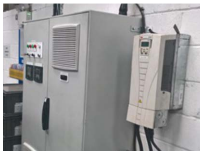
■ Cooling tower controlling panel
